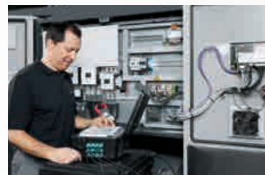
Analysis of compressed air generation
