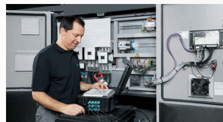
Analysis of compressed air generation
