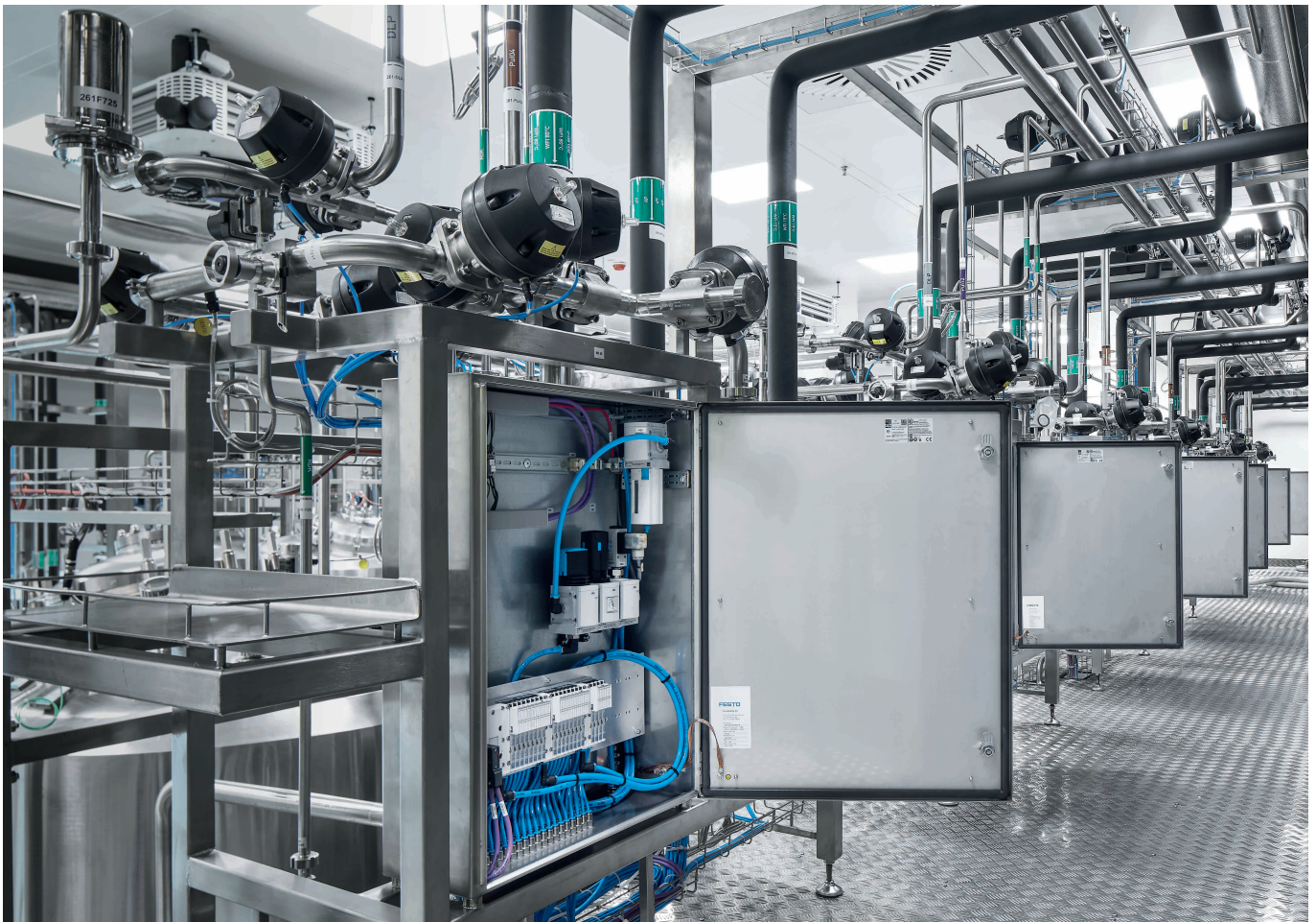
Standardised automation from Festo simplifies installation and maintenance in the large scale plant of Biotest AG.
