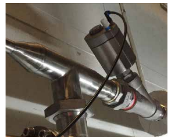
Shut-off control for glycol used in food production
