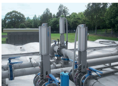
Control of valves in a water treatment plant
